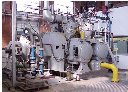
Fig. 1 The Cooper Bessemer GMV-4TF large bore natural gas engine
